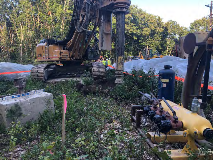
Fig 13: Drill rig at work at Str. 31 with stone walls protected by plastic. Viewing east. (9-13-19).
