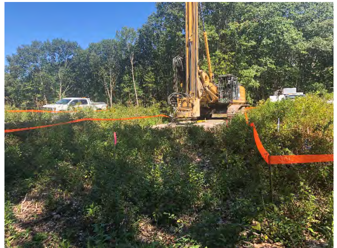
Fig 12: Drill rig setting up for Str. 31 adjacent to stone wall. Viewing west. (9-13-19).
