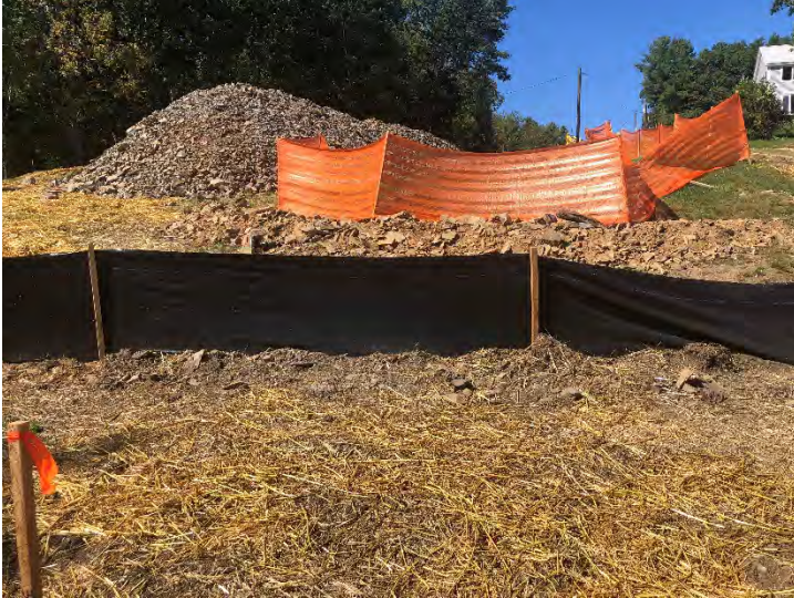
Fig 9: Erosion controls on the eastern extent of Blu Roc trench at Str.99. (9-13-19).
