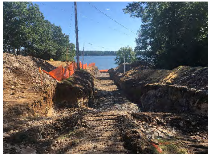
Fig 8: Blu Roc trench on the west side of the Bay. Viewing east. (9-13-19).
