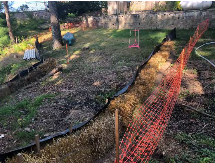
Fig 27: Erosion controls on the east side of the bay. (9-18-19).
