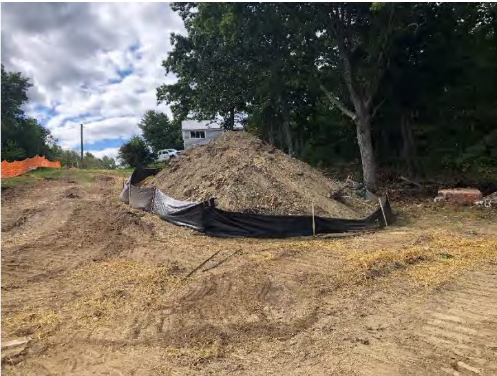
Fig 23: Silt fence downslope from spoil pile at Str. 99. (9-16-19).
