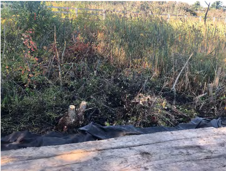
Fig 31: Repaired area of minor soil disturbance in wetland adjacent to matting associated with Str. 131. No additional corrective actions needed. (9-19-19).
